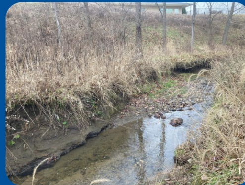
Before: eroding banks adding sediment pollution.
